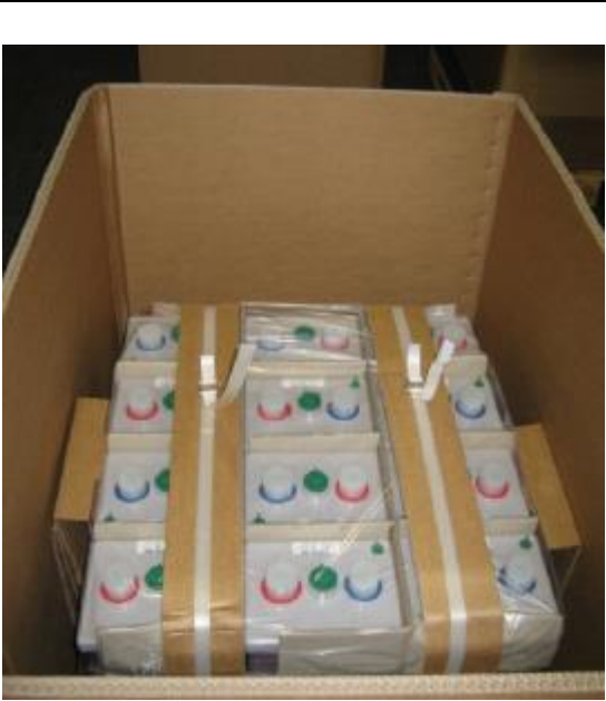
Battery cells with cardboard supports between cells and walls of cardboard box.
